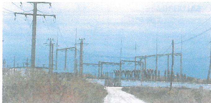
STATIE ELECTRICA - MARUNTISU
